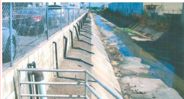
Parking lot designed with these man-made conveyances that connect non-storm water discharges directly to a City drainage channel require a storm drain connection license.
