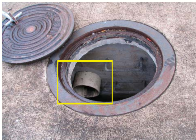
Illegal pipe connection that is below the ground.
