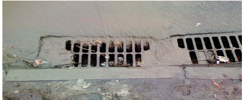
Urban runoff entering a storm drain
