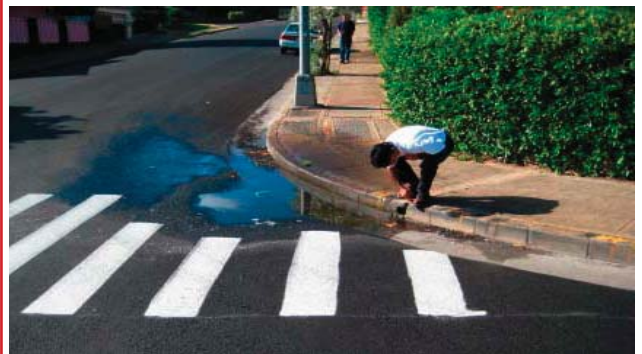
Curb drains typically convey runoff directly to the City's street drainage system without the benefit of absorption by permeable surfaces and natural treatments such as landscaped areas and planters.
