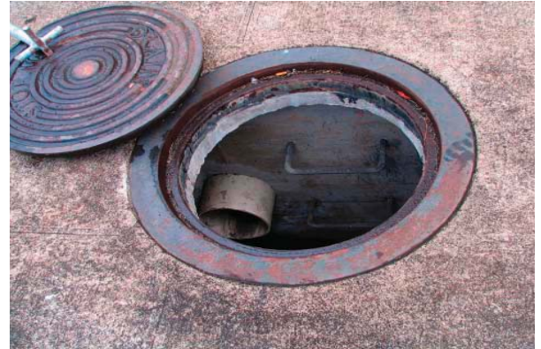
Illegal pipe connection that is below the ground
