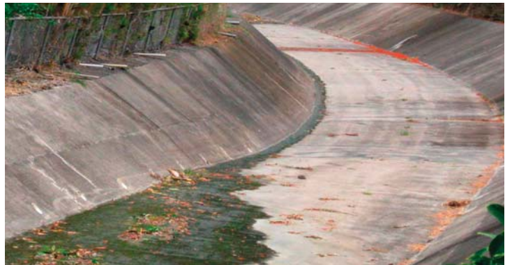
Each pipe is a man-made conveyance that connects non-storm water discharges directly to the city-owned separate storm sewer system or MS4. Illegal connections can be located either above or below the ground and may include drains, pipes or ditches.
