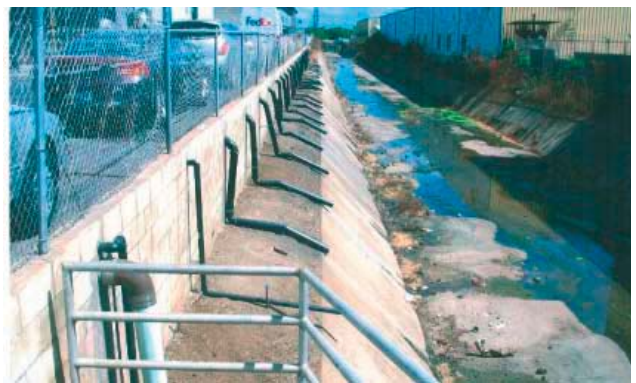
Parking lot designed with these man-made conveyances that connect non-storm water discharges directly to a City drainage channel require a storm connection license.
