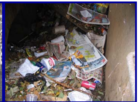
Trash inside a catch basin
