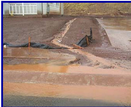
Soil erosion during construction
