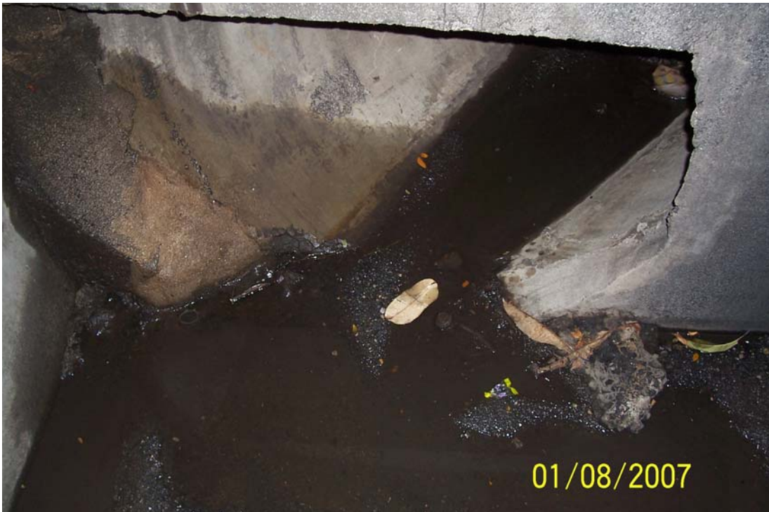
Possible illegal discharge
