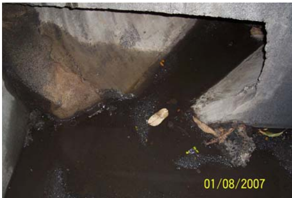
Possible illegal discharge
