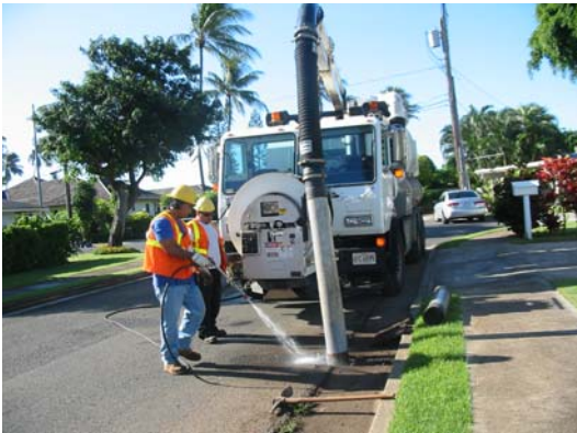
Clogged inlet in residential area
